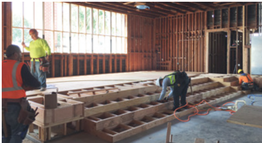
A permanent stage is being constructed to showcase the talents of Hutchinson's wonderful Choir, Band & Orchestra students.
